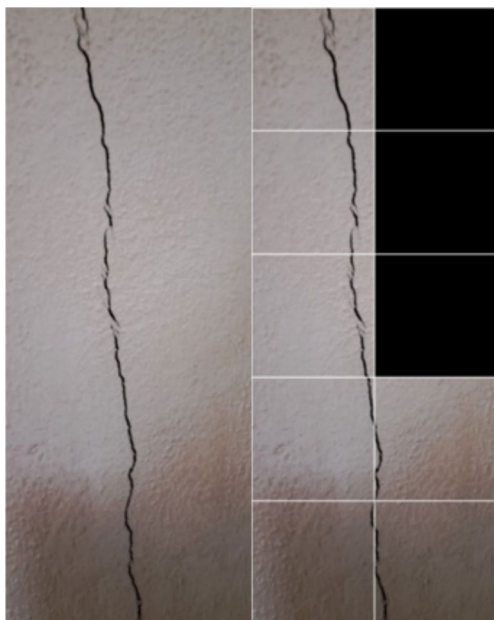
Fig. 15 Concrete image (on the left) and the corresponding image classified in crack patches and non-crack one, the latter represented in black (on the right)
